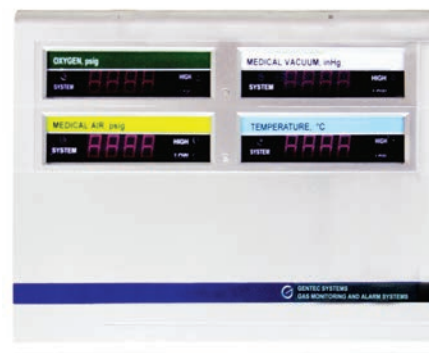
Area Alarm with Local Sensors
